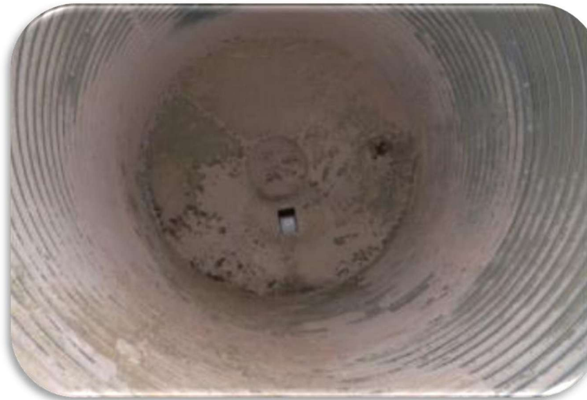
✓ Siloz murdar, contaminat
